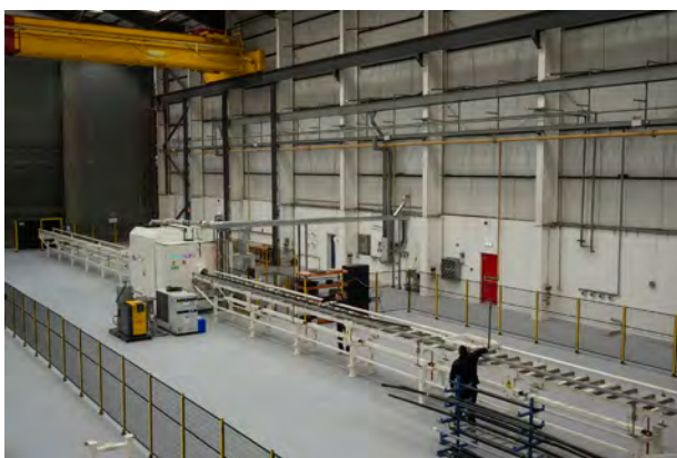
Figure 5. An Enoflex laser-welding station contained within a light-proof box. Roller-tracks feed the pipe into the welding station for example from reeling carousels.
